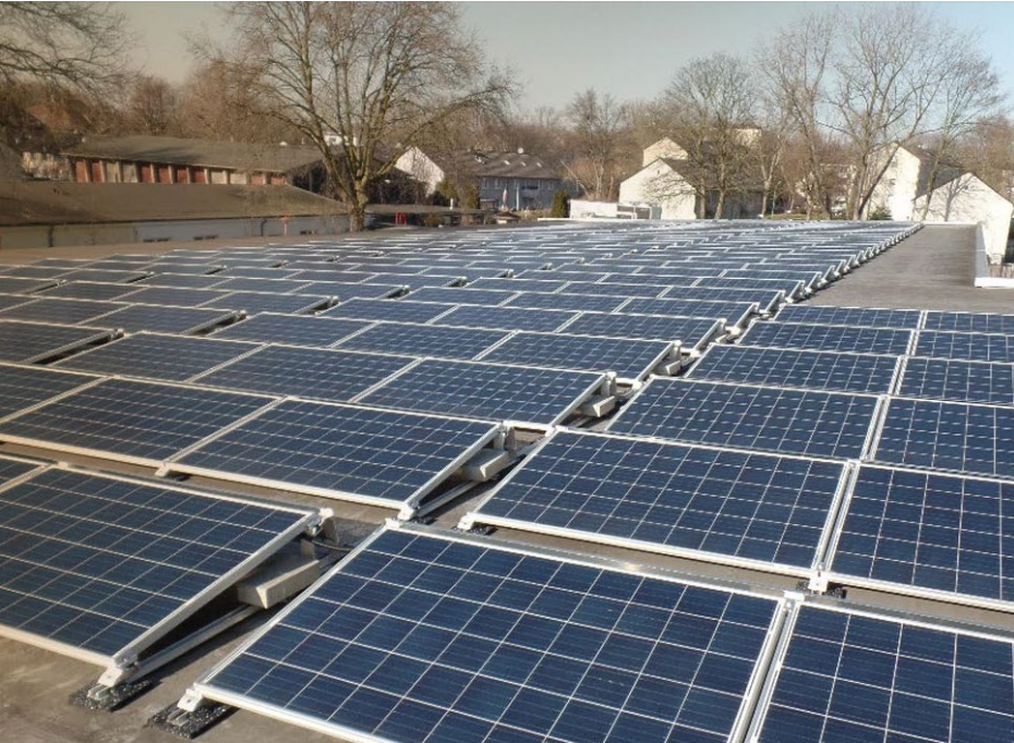
PV roof system
