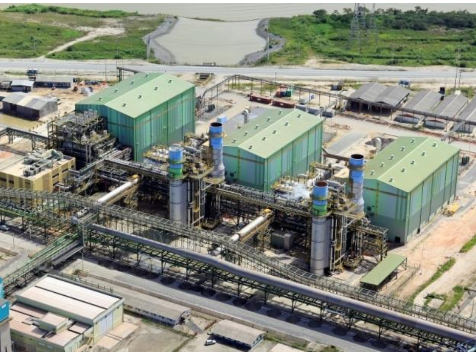
Atlantic steel power plant (490 MW), Sepetiba, Brazil
